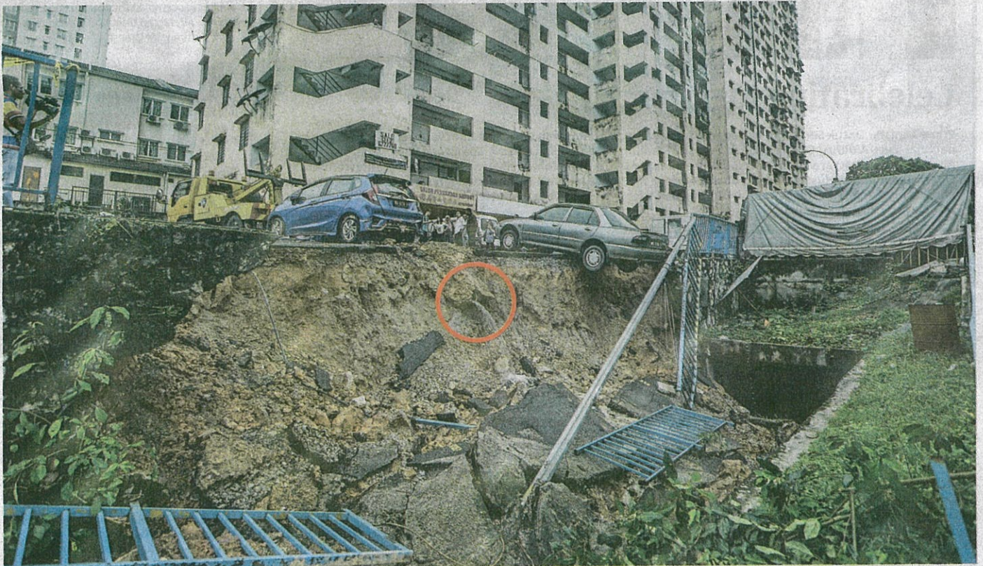
Erosion caused by the collapsed drain pipe (circled). — Picture by Hari Anggara
