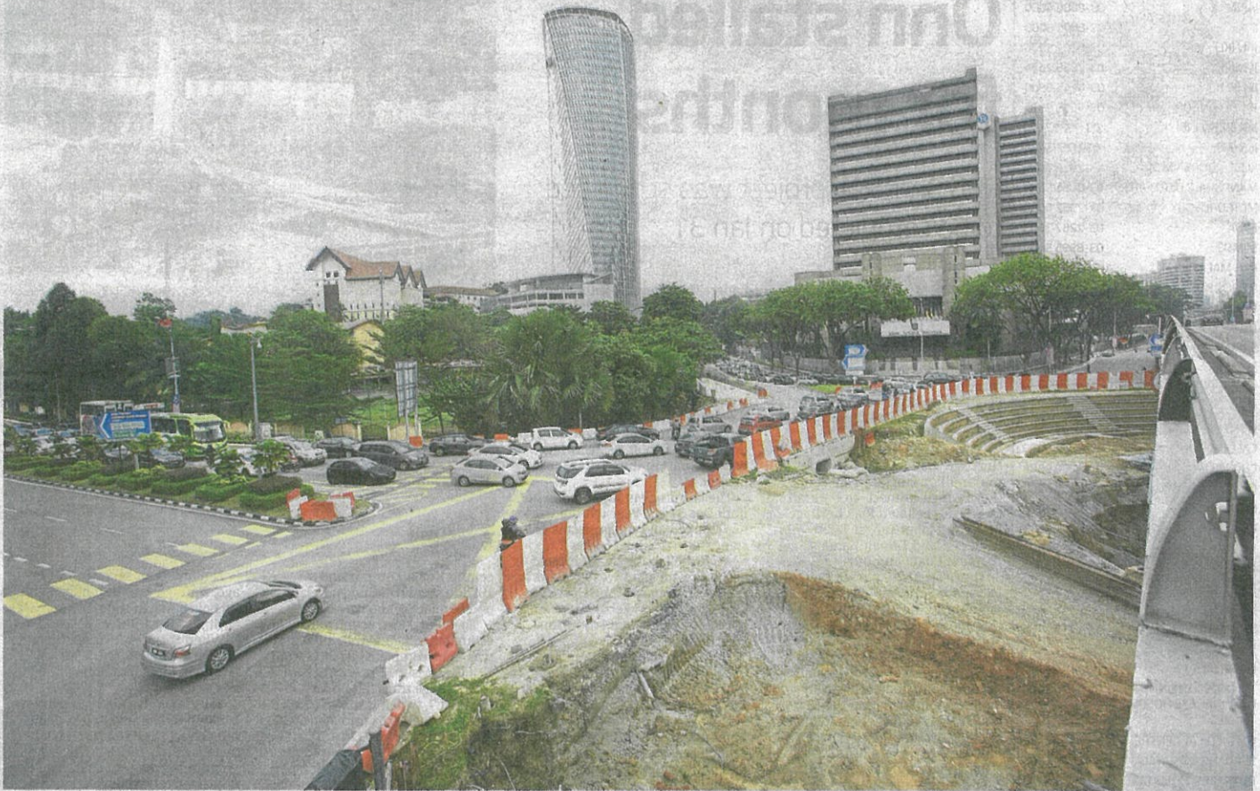
Stumbling block: The abandoned project site at Bulatan Dato' Onn is an eyesore and the prolonged road closure is an inconvenience to motorists. — IZZRAFIQ ALIAS/The Star
