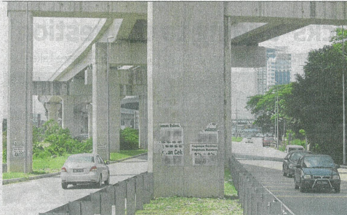
Illegal advertisements pasted on the pillars of the LRT Bandar Puteri station along Jalan Puchong.
