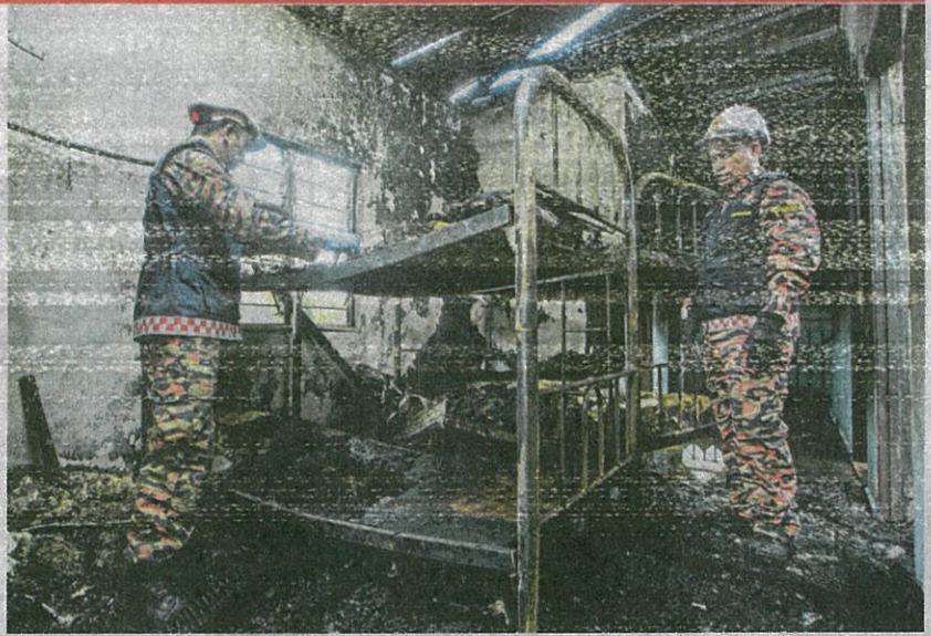
Fire and Rescue Department personnel inspecting the damaged building of the Nur Al-Quran Learning and Tahfiz Centre in Kapar, Klang, yesterday. PIC BY MUHAMMAD SULAIMAN
