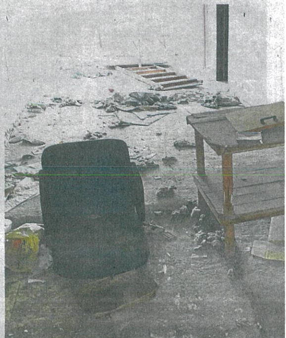
Furniture scattered in the corridors of the unfinished Bukit Rimau Indah flats project.
