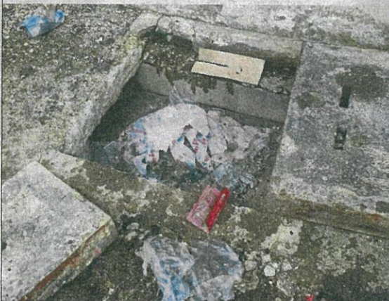
The drains in the backlane of Jalan Setia Indah X U13/X are clogged with food waste dumped by errant restaurant operators.
