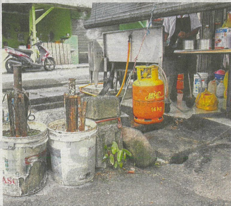
This hydrant in Taman Indah, Cheras, is barely noticeable as the paint has faded and it is blocked by other objects. Under the Service Act and Regulations 1988, it is an offence to cover up, enclose or conceal any fire hydrant or to use it for any reason other than fire-fighting purposes.
