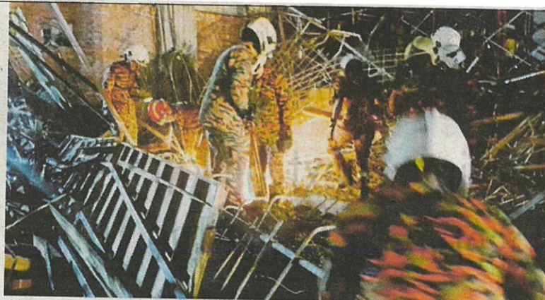
City Fire and Rescue Department personnel recovering the body of a Bangladeshi worker at a building project site in Jalan Cochrane, Kuala Lumpur, yesterday.
