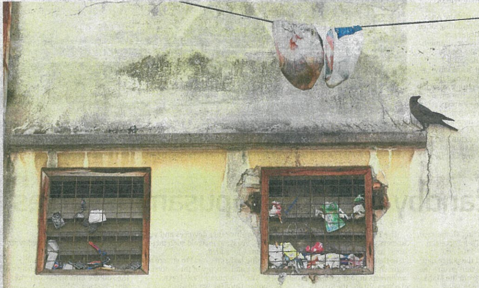
A bag filled with rubbish hangs from cable at a flat in Bukit Bintang. Rubbish is also trapped in the window panes.
