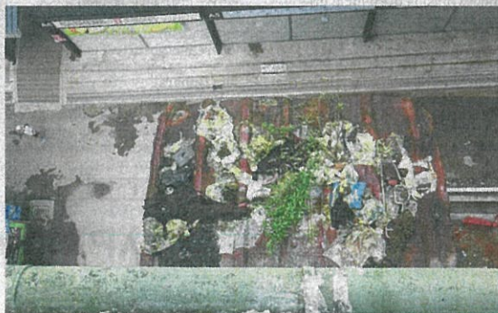
A view from above showing rotting rubbish on an awning.
