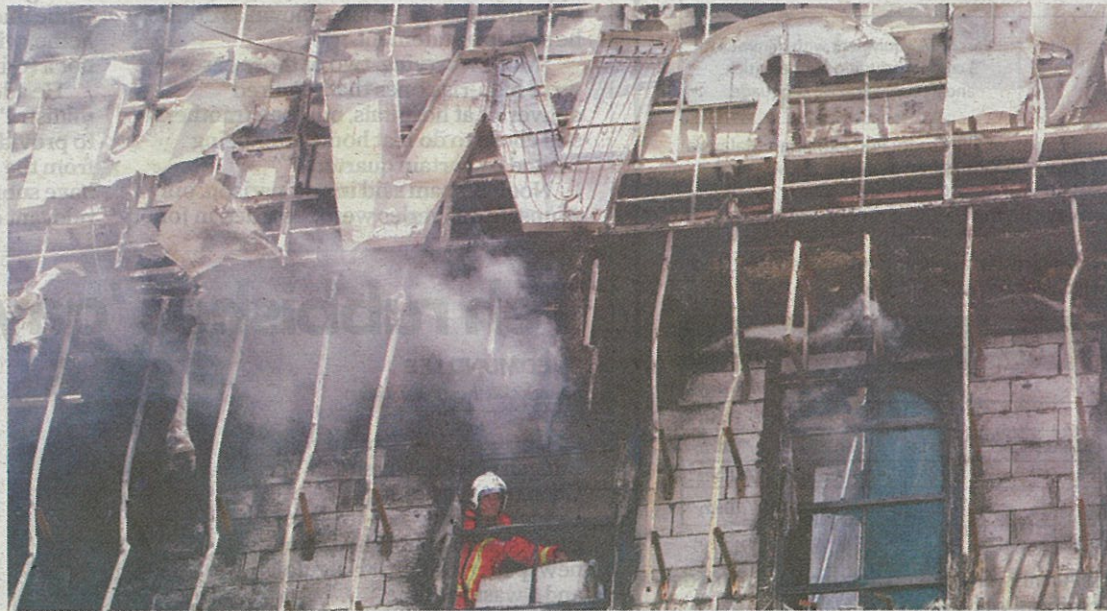
A firefighter checking the damage after the fire yesterday.
