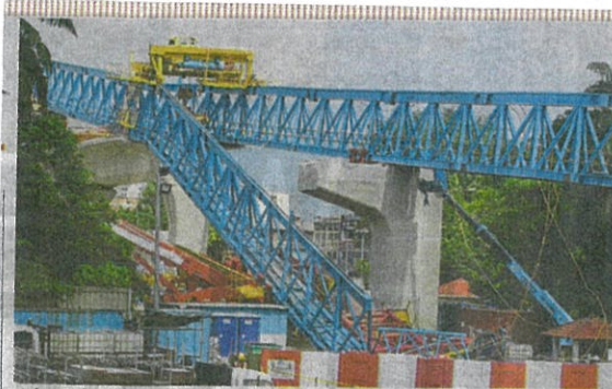
A launching gantry collapsed at a Mass Rapid Transit construction site in Kuala Lumpur on Saturday. PIC BY MOHD YUSNI ARIFFIN
