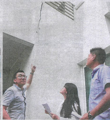
(From left) Tiew, Wong and So inspecting a cracked wall.
