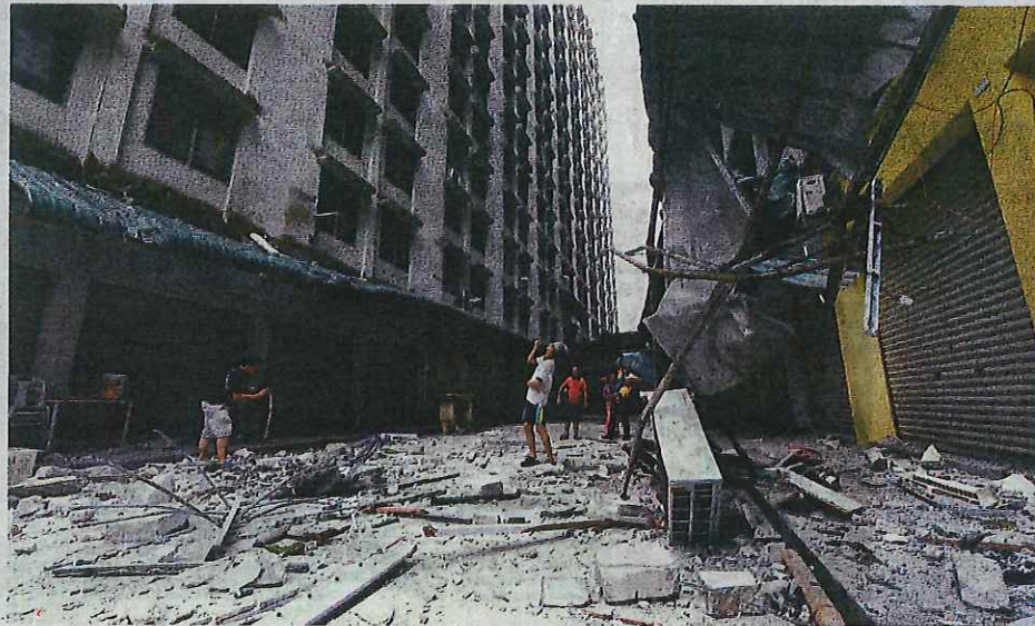
Desa Green residents walk through the rubble yesterday. —BERNAMAPIX
