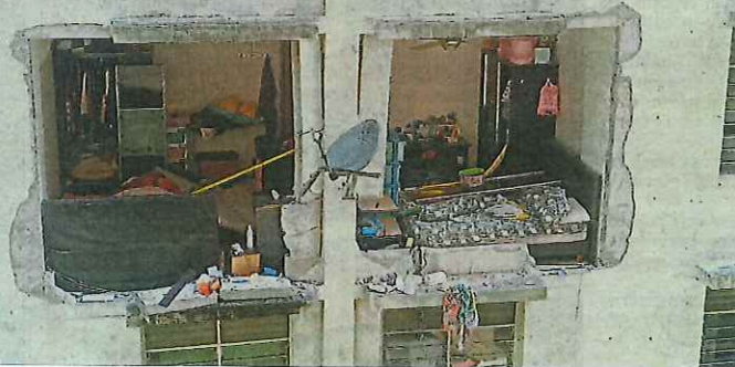
Devastation: The Bomba Forensics team visiting the site of the blast to collect samples. (Left) Walls from the Green Garden apartment unit after the blast that killed a 62-year-old man.
