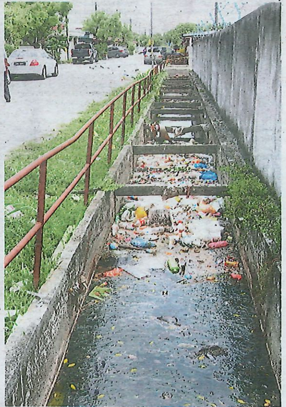
Rubbish clogging monsoon drains in Klang. Residents want the contractors appointed by MPK to do their jobs properly. — Filepic
