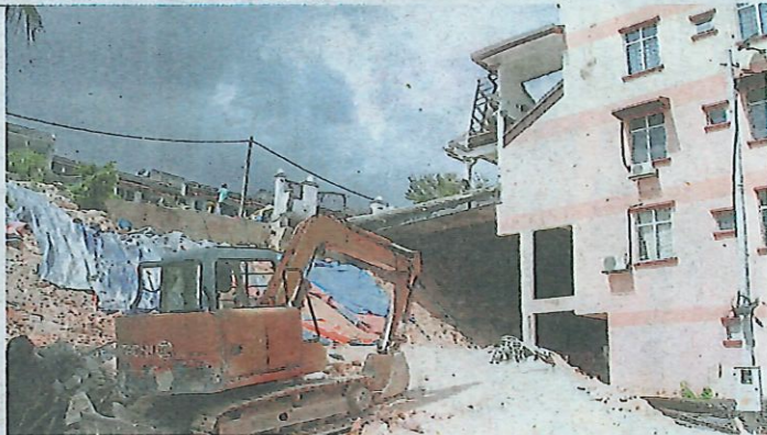
Repair works at Taman Lagenda Mas, Jalan Mas 11, in Cheras due to a landslide. - Filepic
