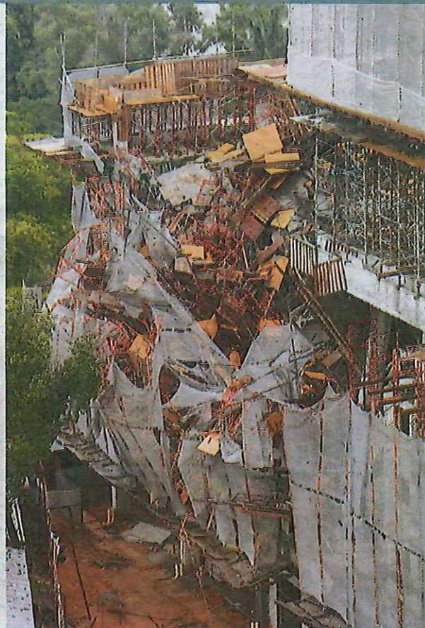
A section of the affected structure in Taman Desa, Kuala Lumpur. —BERNAMAPIX
